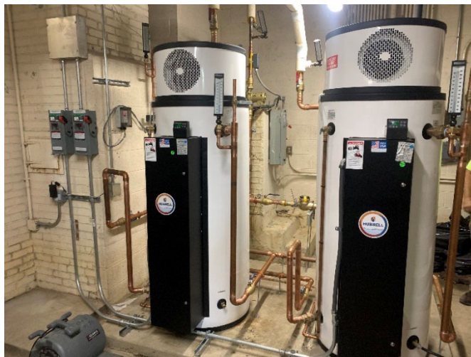
Figure 5. Heat pump water heaters for Lee Center electrification
